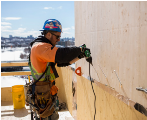
Balloon-frame system allows work to be completed at the height of man © Photo: Stéphane Groleau
