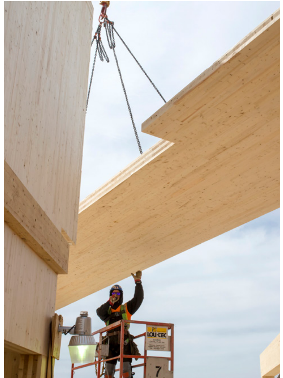
Installing a floor slab, a small portion of which will come to rest on the wall plate attached to the left wall © Photo: Stéphane Groleau
