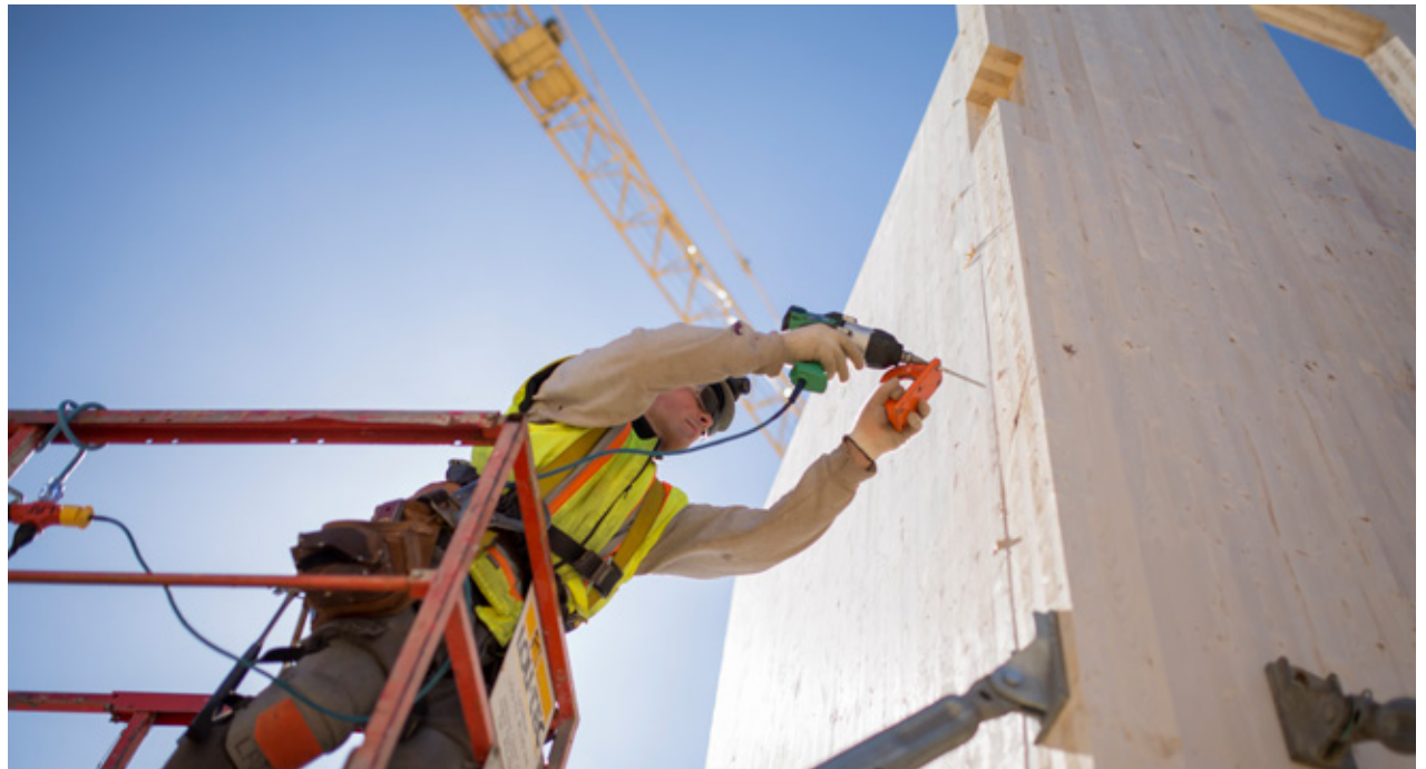
Lifting fitting are removed after the installation of CLT panel © Photo: Stéphane Groleau
