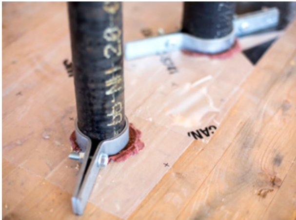
Red caulk ensuring the degree of fire separation around equipment passing through a CLT panel © Photo: Stéphane Groleau
