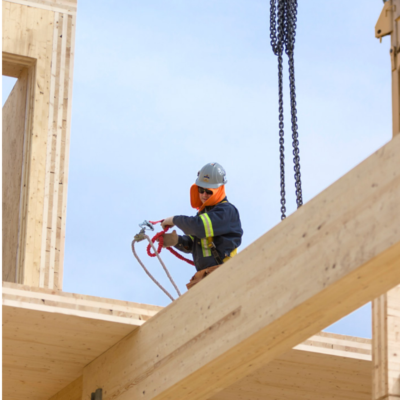
Wood elements arrive on site with all cutouts and openings pre-cut © Photo: Stéphane Groleau
