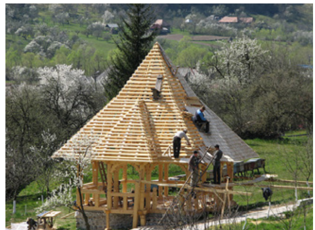
One of the smaller churches under repair showing the type of wood construction used in all of the monastery structures.
