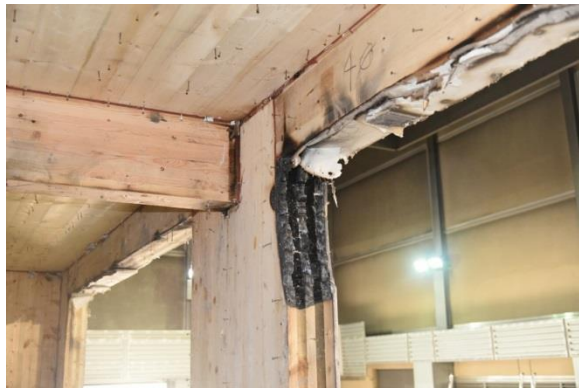
e) damage at second floor window
