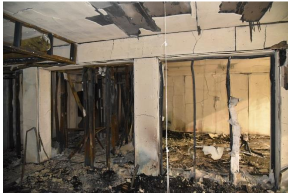
a) Compartment after Test 1
