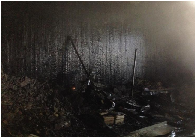
c) Charring of side wall
