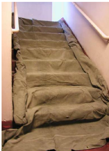
Figure 13. Use of salvage cover to protect and divert water down stairway [67]
