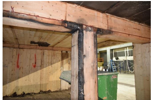
d) Damaged column and beam
