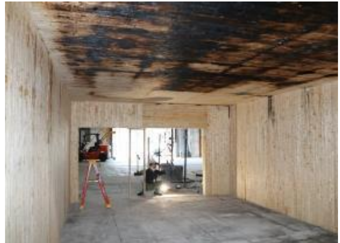
b) Test 1-2 condition of CLT after test
