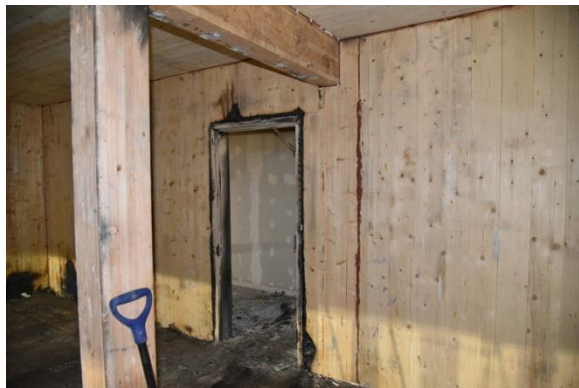
g) damage around apartment door
