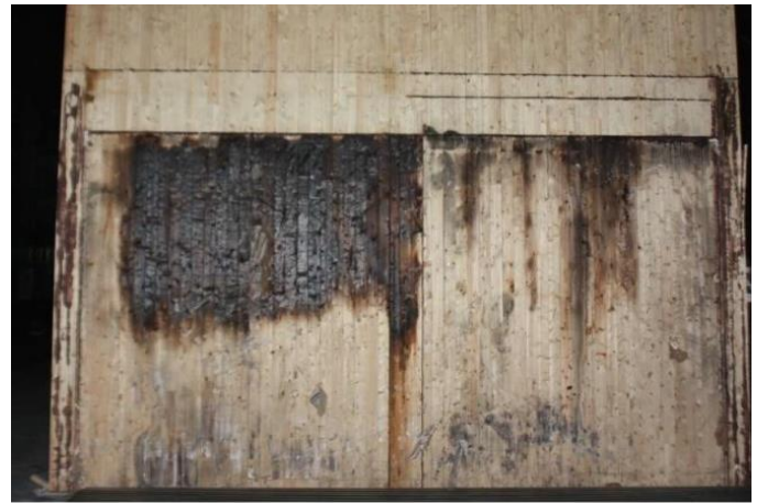
d) Condition of shared wall after test (NRC)
