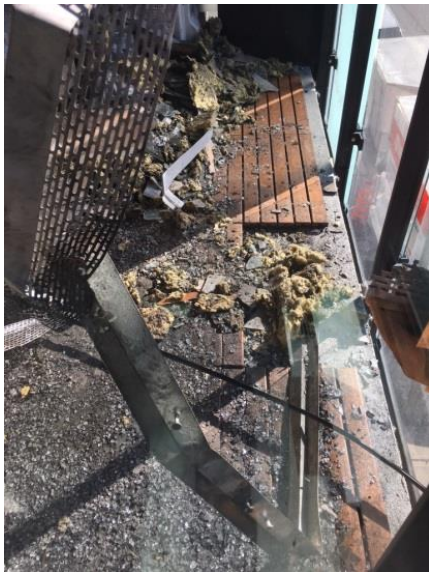
c) Balcony damage
