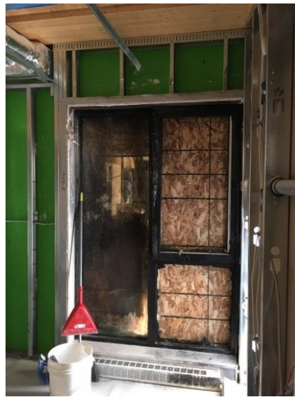
d) Damage to opening from interior
