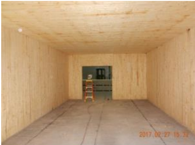
a) Test 1-1 compartment after test
