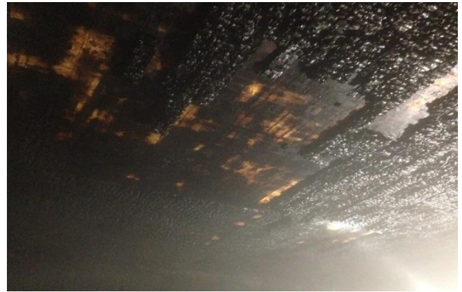
b) Charring of ceiling. Some 2nd CLT layer in place, 3rd layer exposed
