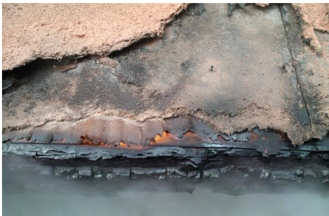
e) Charring at window opening, evidence of uncharred wood beneath gypsum
