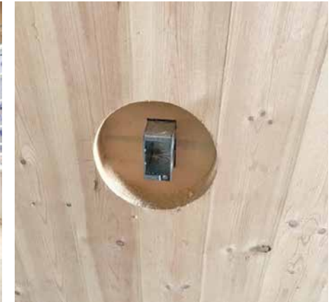
6.9 A circular hole for a square receptacle requires a custom cover plate
