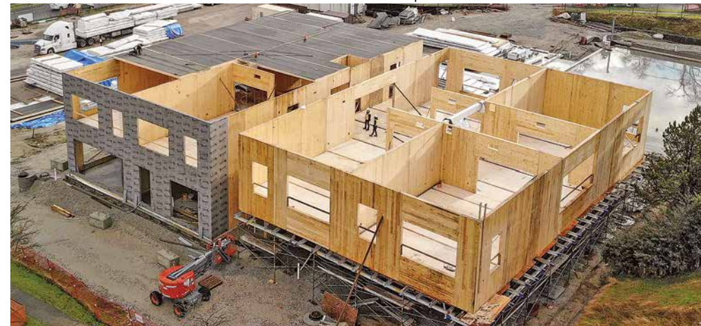
6.10 The double cantilever is supported by projecting CLT walls reinforced with steel
