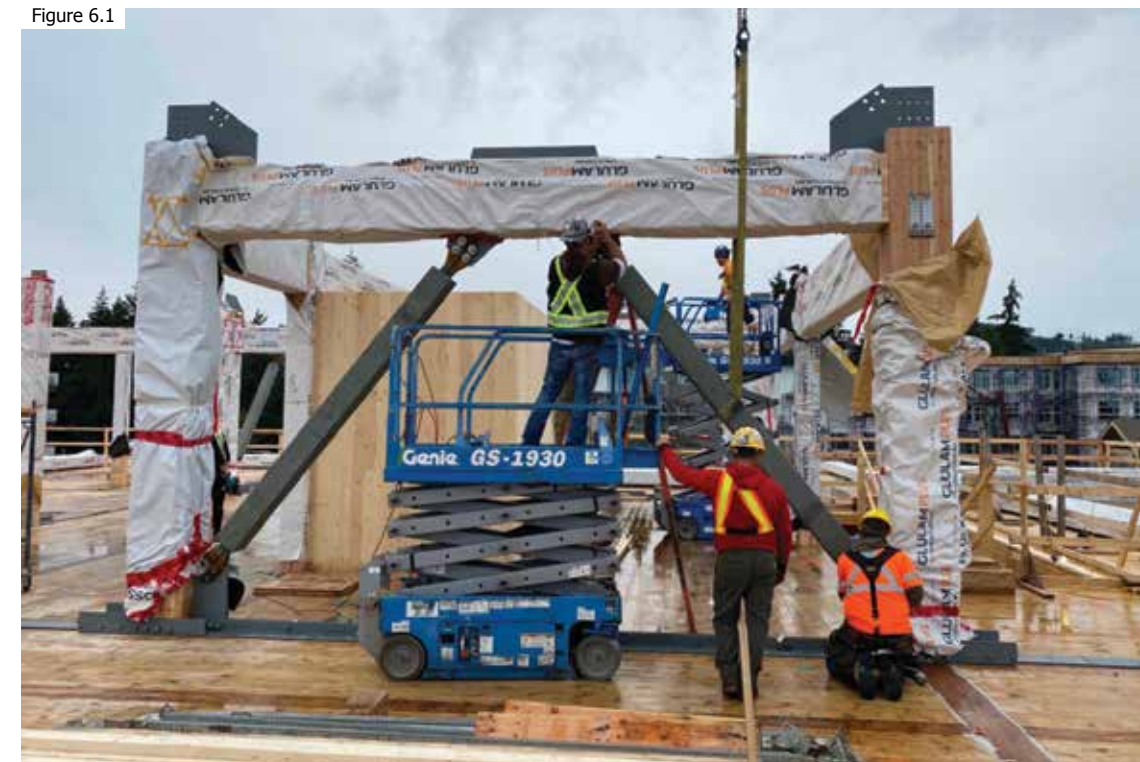
Figure 6.1: Factory installation of the base connections ensured that field installation of the bRBs would be straightforward. (Credit Aspect Structural engineers)
